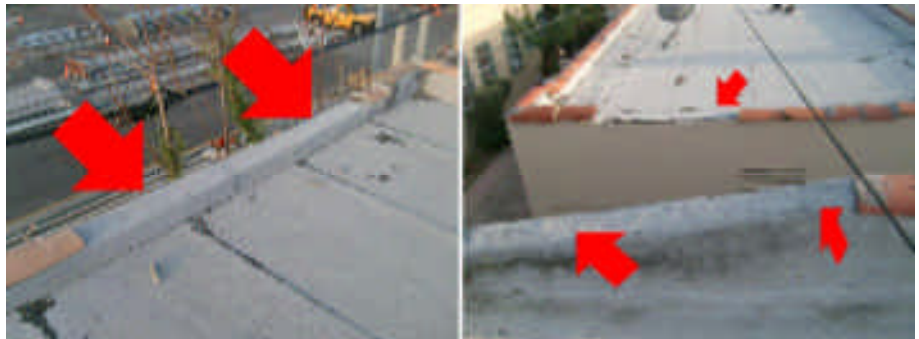
There are many tiles missing along the parapet walls.
