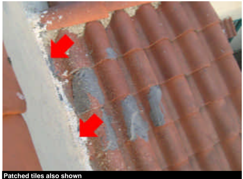
Patched tiles also shown
