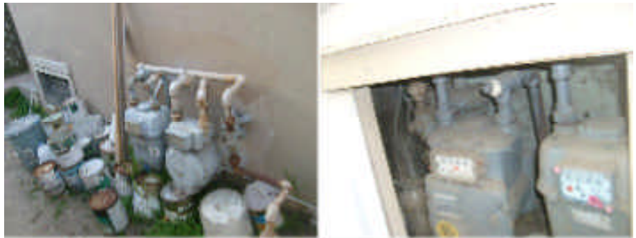
The gas meters are located around the outside of each building.
