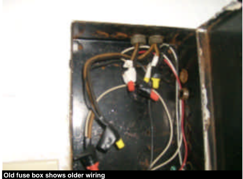
Old fuse box shows older wiring
