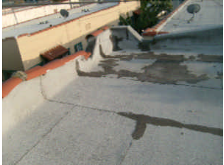
The back left duplex has areas of worn granules and many patched areas.
