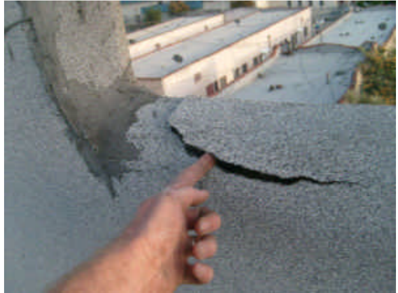
There is a torn cap sheet along the front edge of the back building.
