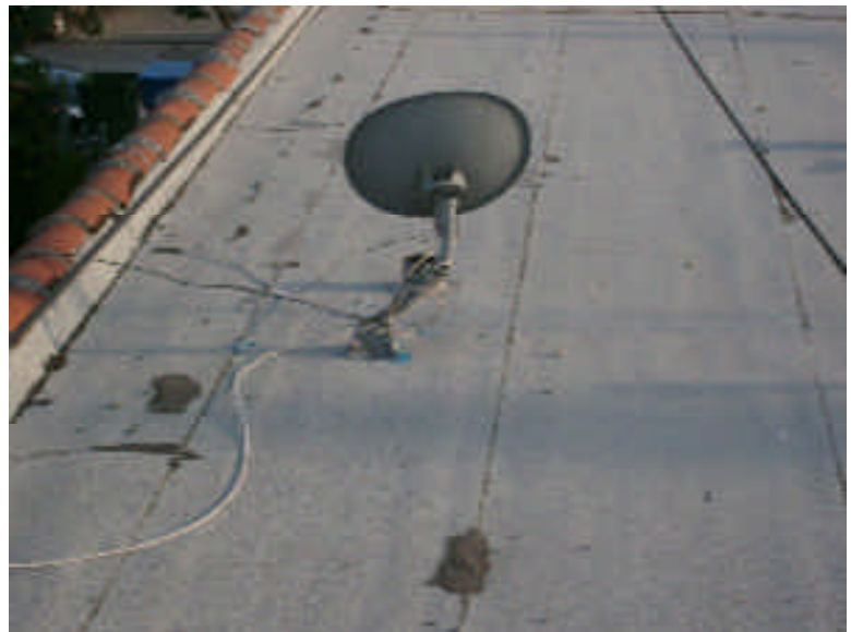
Needs Attention:;, some of the TV satellite dishes are mounted directly down screwed into the roofing material;
